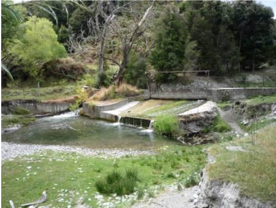
Water diversion structure in Quartz Creek
