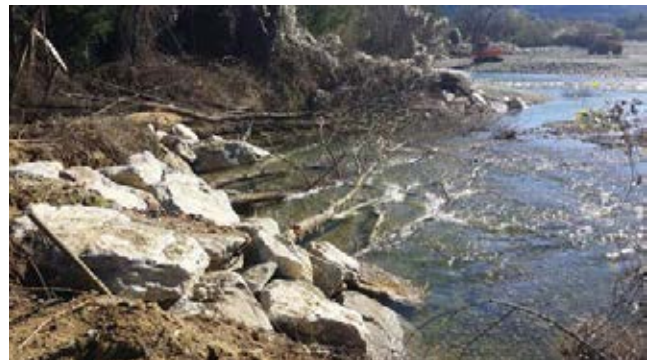
^ TDC are now using rock groynes with live willows anchored to provide future shading and bank stabilisation
